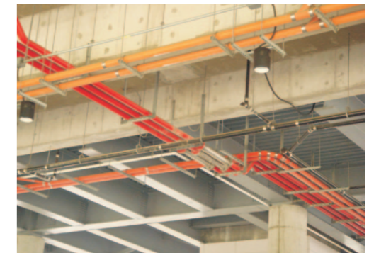
消防管 Fire Services Pipe
