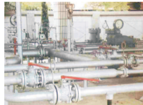
瓦斯壓力配管 Gas Pressure Services
