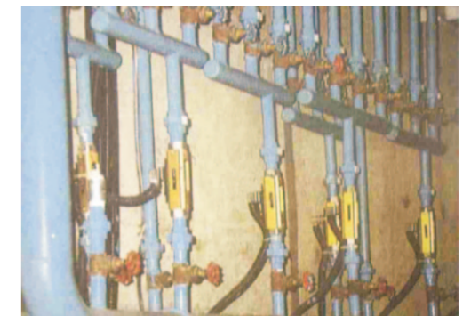
冷凍管 / 空調管 Refrigeration/Air-conditioning Pipe
